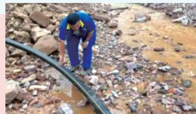
The rescue team of Songxian Company conducts an on-site inspection and formulate a rescue plan after the buried medium-pressure gas pipeline was swept away by the river
